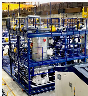
Gas Treatment Unit UPG-02-57000-4.0-KhL1
